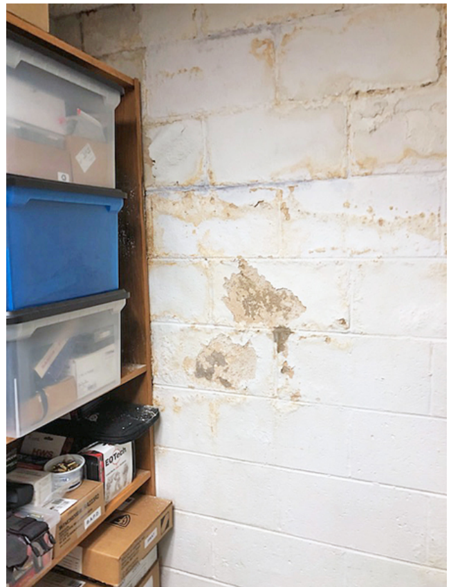
Water and mold permeate most spaces in the current station.
