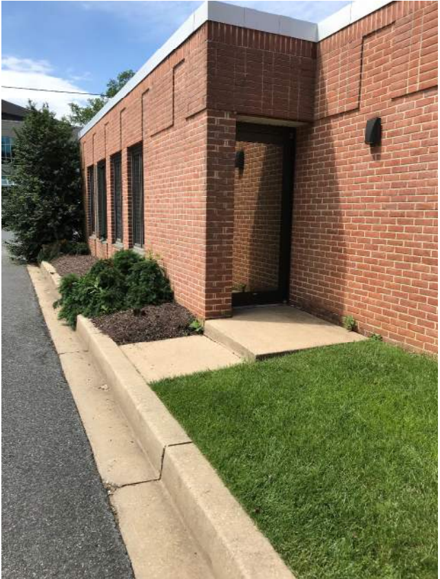
Non-ADA Accessible Exit
