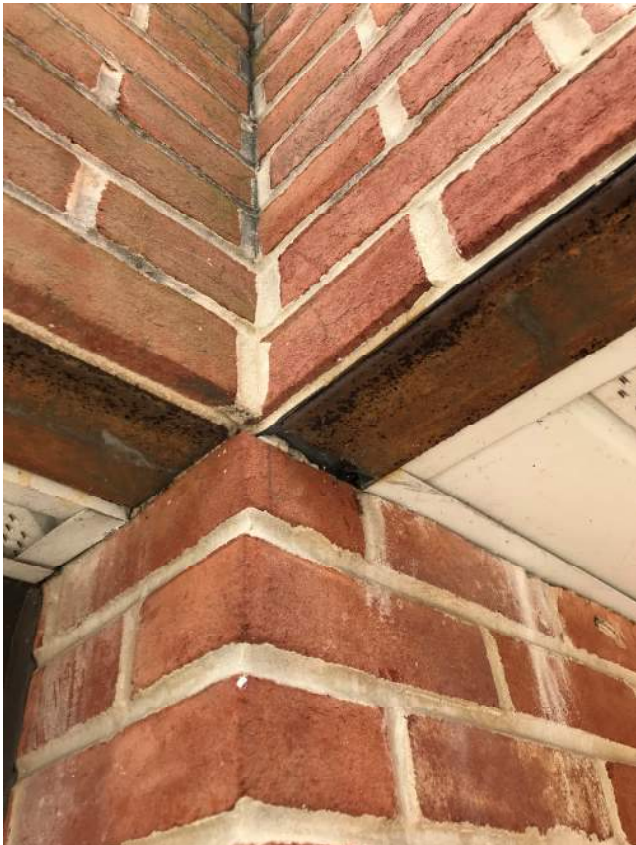
Steel Support Lintel Deterioration
