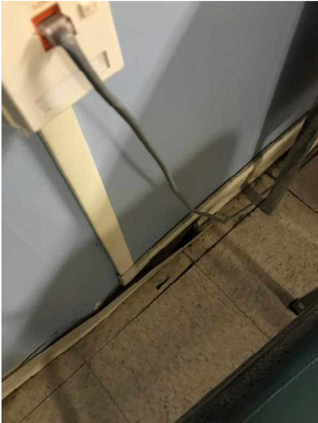
Deteriorated/Damaged Wall and Base
