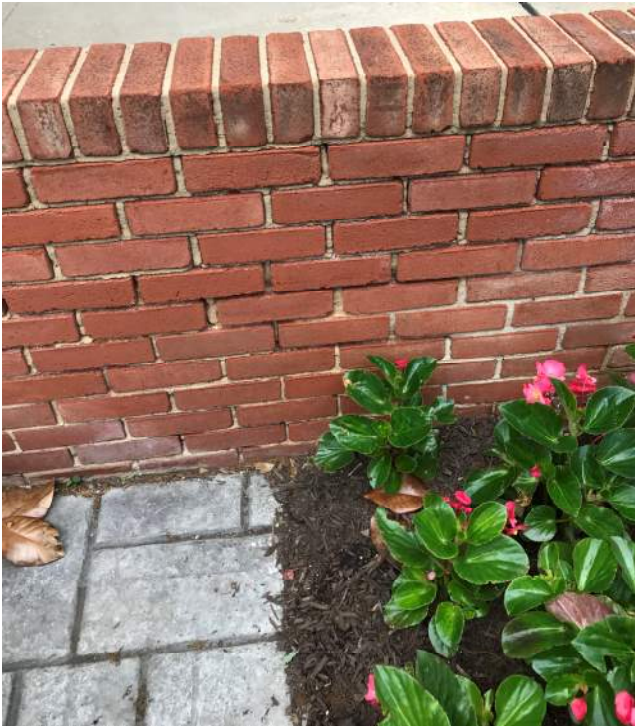
Deteriorated Masonry Retaining Wall
