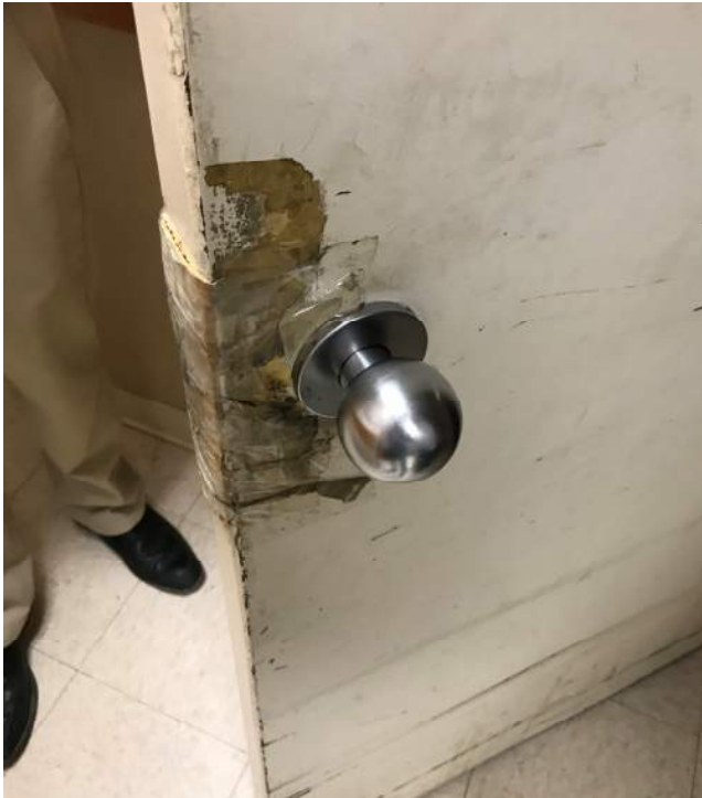
Damaged Door and Hardware
