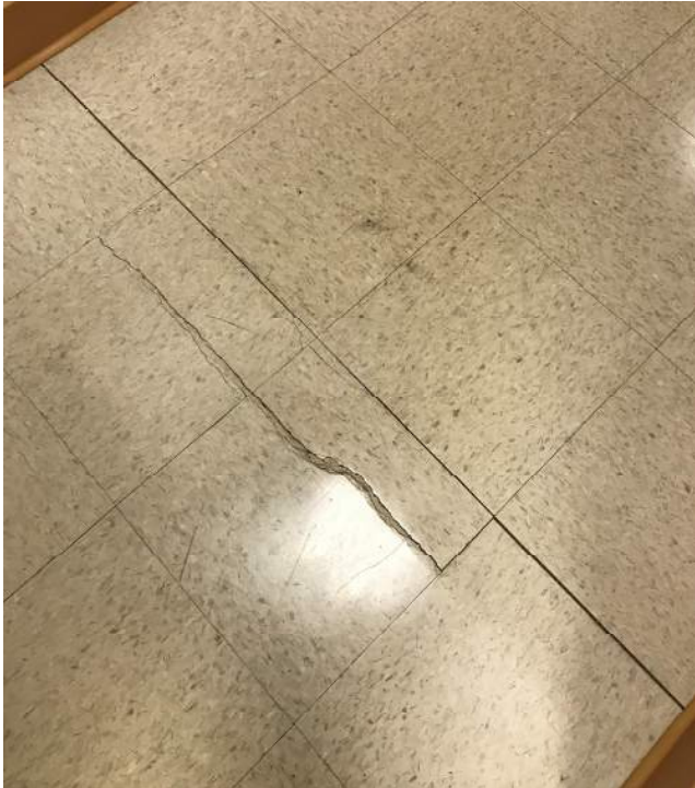
Deteriorated/Damaged Floor Tile
