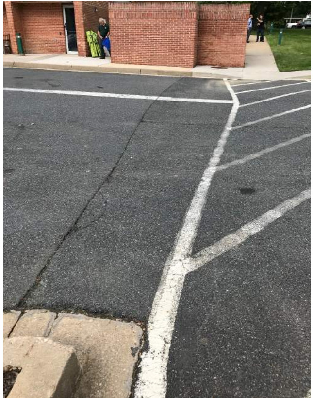
Deteriorated Macadam Driveway
