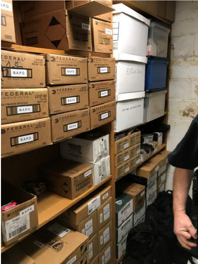
Damaged CMU Wall and Finish
