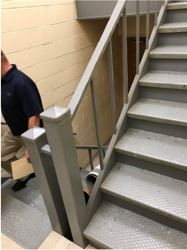
Non-Code Compliant Stair Railings/Guardrails
