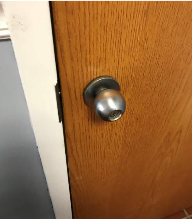
Non-ADA Accessible Door Hardware
