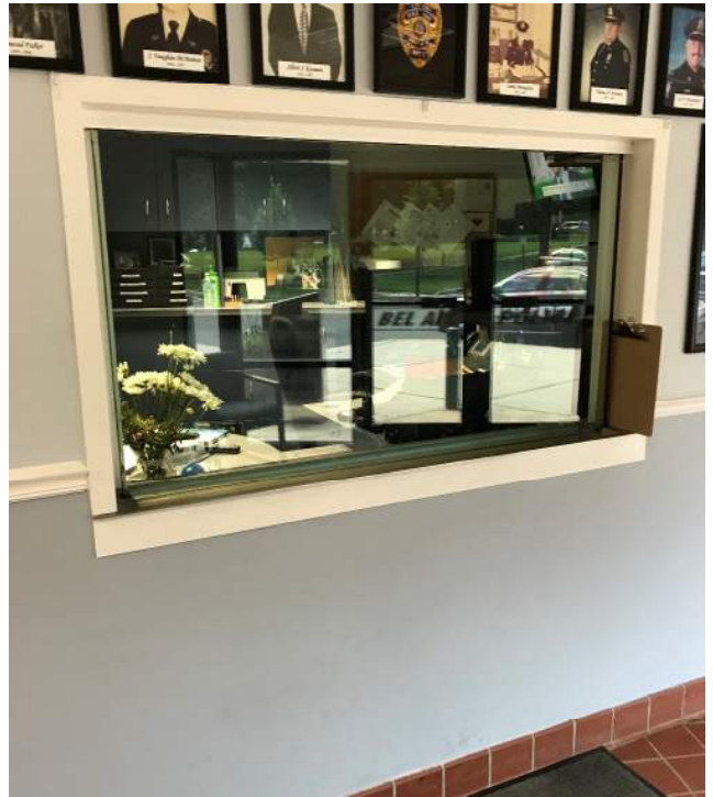
Non-ADA Accessible Main Reception Window
