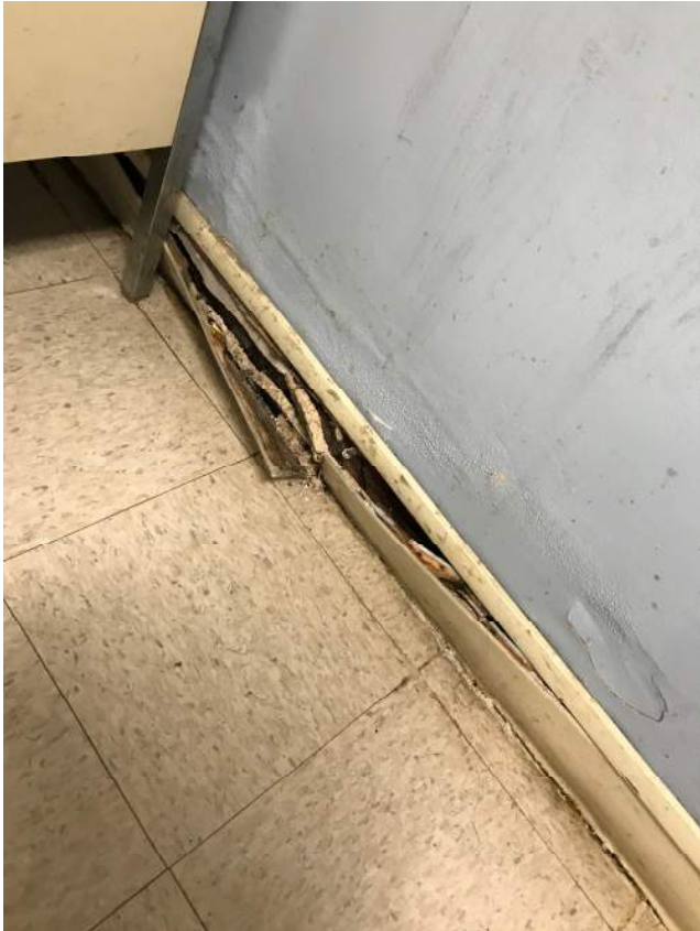
Deteriorated/Damaged Wall and Base
