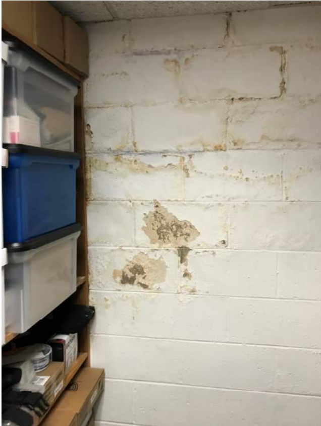
Damaged CMU Wall and Finish
