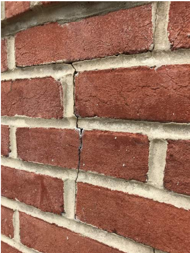
Deteriorated Masonry Wall
