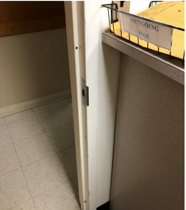
Non-ADA Accessible Door Approach
