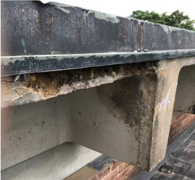
Deteriorated Concrete Roof Structure
