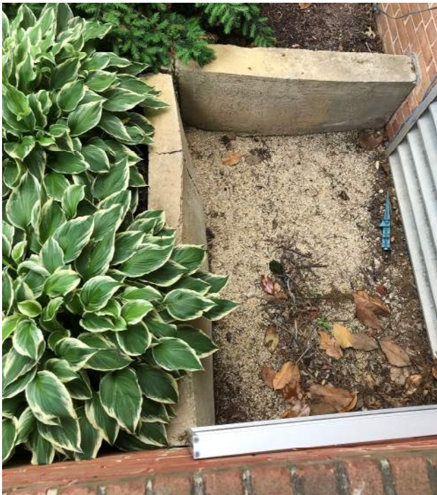
Deteriorated Concrete Areaway
