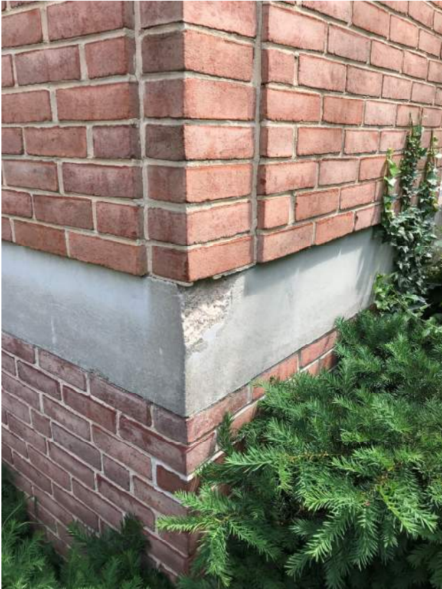
Deteriorated Concrete Banding
