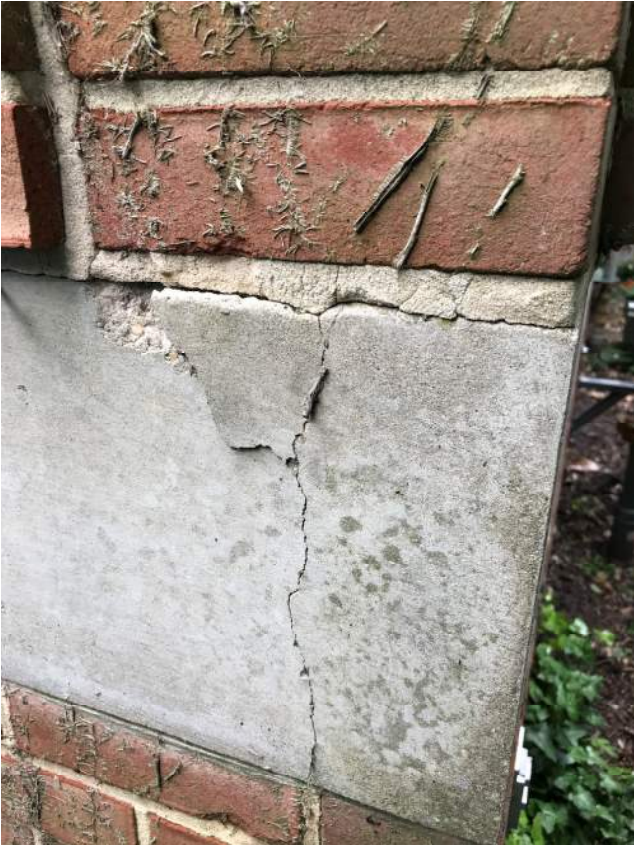
Deteriorated Concrete Banding
