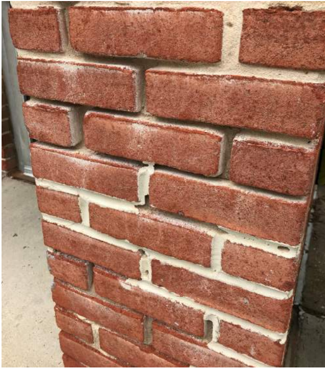
Deteriorated Masonry Wall
