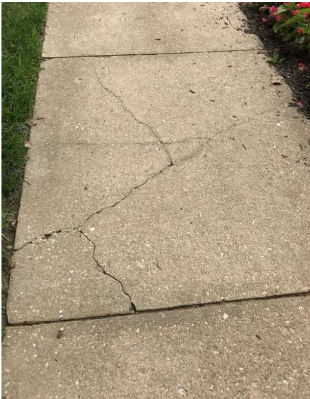
Deteriorated Concrete Walkways
