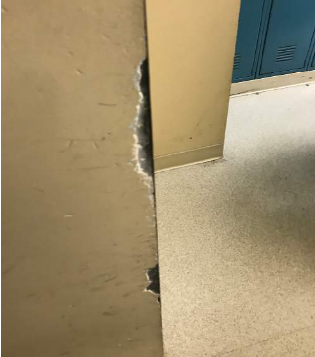
Damaged Wall Finish
