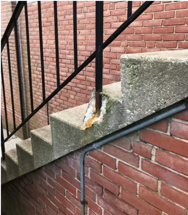
Deteriorated Exterior Stairs
