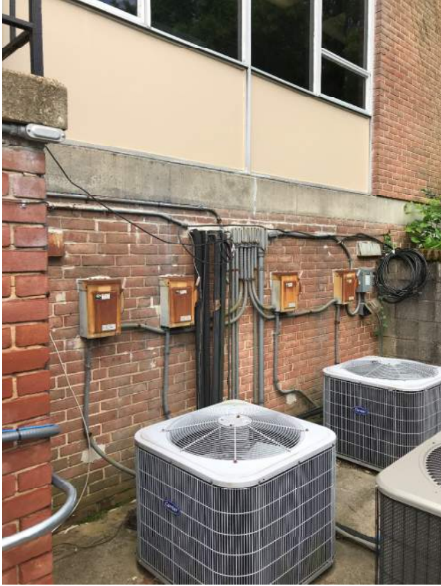
Exterior HVAC Service
