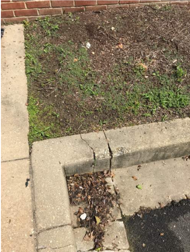
Deteriorated Concrete Curbing
