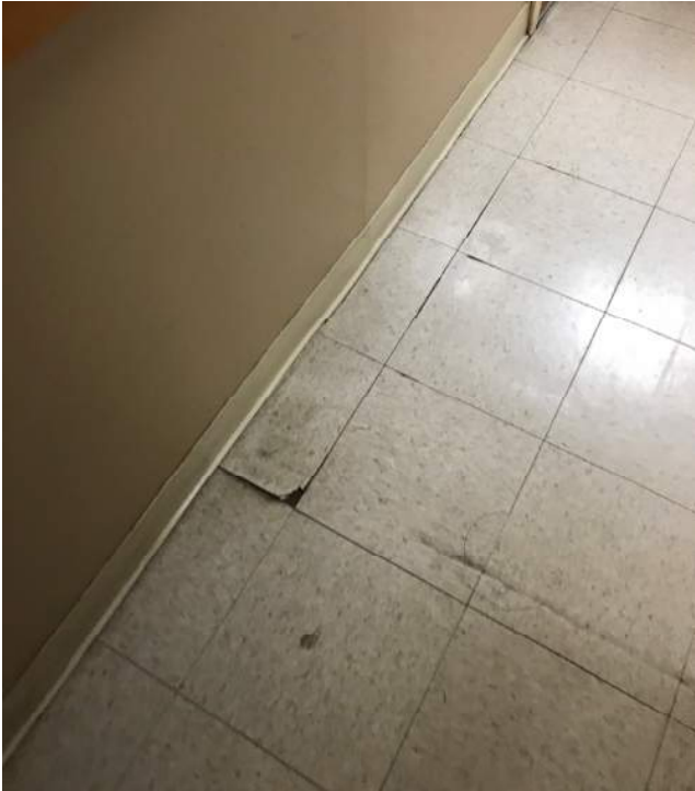
Deteriorated/Damaged Floor Tile
