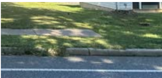
Incomplete sidewalk on Rock Spring Road
