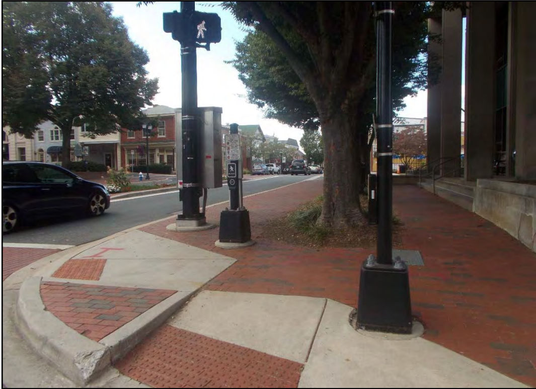
Figure 9. Ramps With Full-Height Curbs Creating Tripping Hazard
