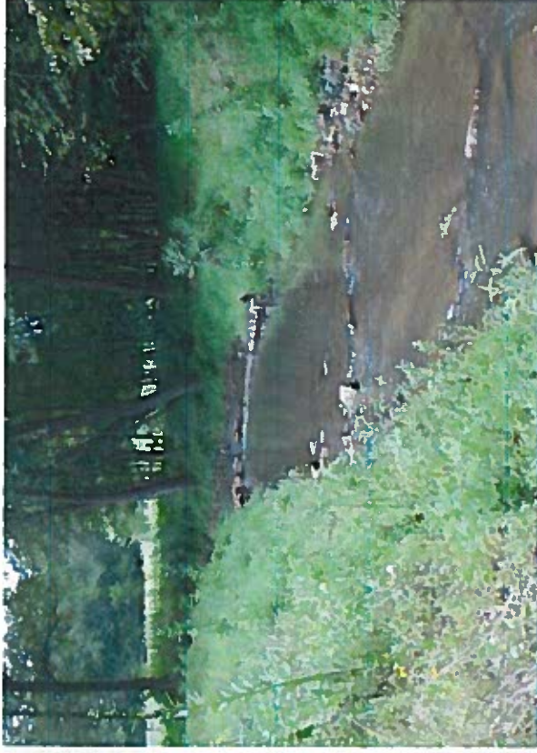
(b) Same reach one year after restoration. Note channel narrowed and constructed riffle and log-boulder J-Hook installed to provide vertical and lateral control
